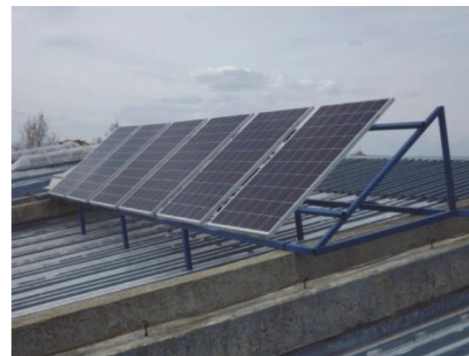
Fig. 1. PV solar power plant, 1.05 kW p
