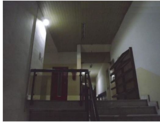
Fig. 4. Solar lighting inside the Faculty
