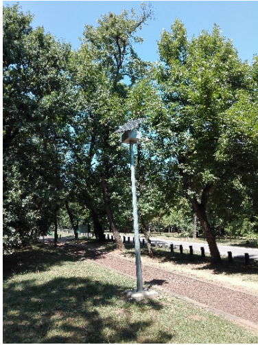
Fig. 5. Lighting column with solar module
